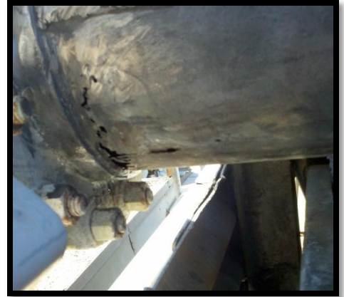
View of Thru wall defects
